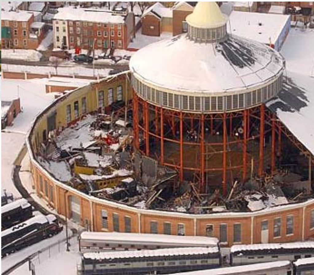
17th February 2003 – Collapse due to heavy snow storm unbalanced load on half roof
