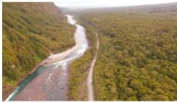
Road exposed to river erosion
