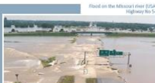
Flood on the Missouri river (USA), Highway No 54.
