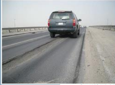
Pavement deformation by hot temperature and overload
