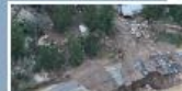
Road damaged by river erosion and simultaneously by mud from the transversal valley
