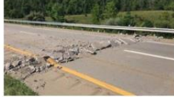
Hot weather causes concrete to buckle
