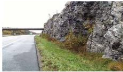
Unprotected rock cut very close to the road
