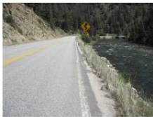
Road exposed to river erosion
