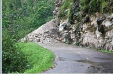
Massive rock fall from the unprotected rock slope
