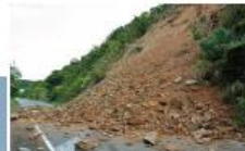
Massive landslide from an unprotected slope
