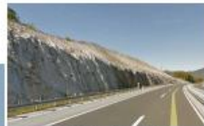
Road cut on the rocky way without any treatment of the rocks and eroded slope
