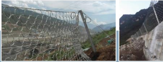
Debris flow barriers
