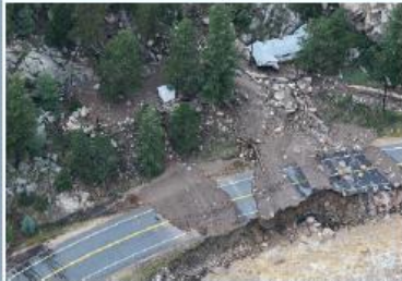
Road destroyed by river erosion and subsequently by heat from the transversal valley
