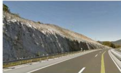
Cut on the motorway without any treatment of the rocks and eroded slope
