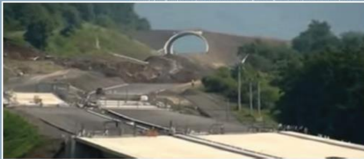
Landslide on the D8 motorway detached section between bridge (under construction) and tunnels for animals' migration. Motorway opening delayed for 3 weeks. Costs of rehabilitation grew during works; railway track was not reopened till now.
