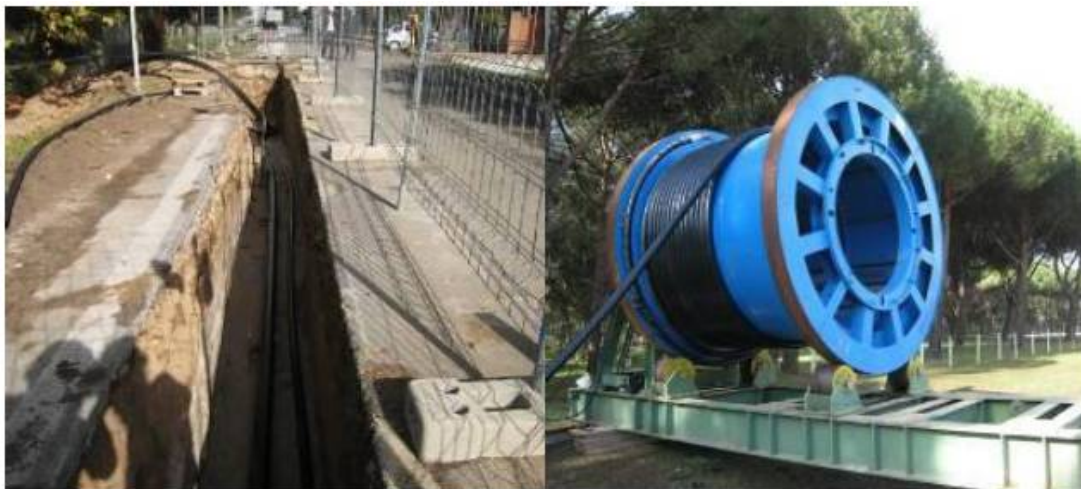
pic.25. trench example and typical coil for underground cable
