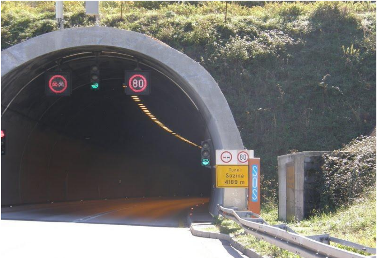
Figure 3.5: ITS equipment in the Sozina Tunnel
