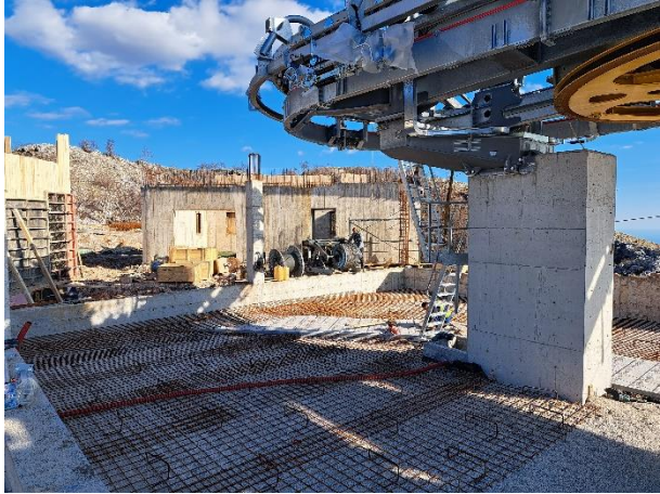
Figure 10-4: Top station / start of the rope assembly
