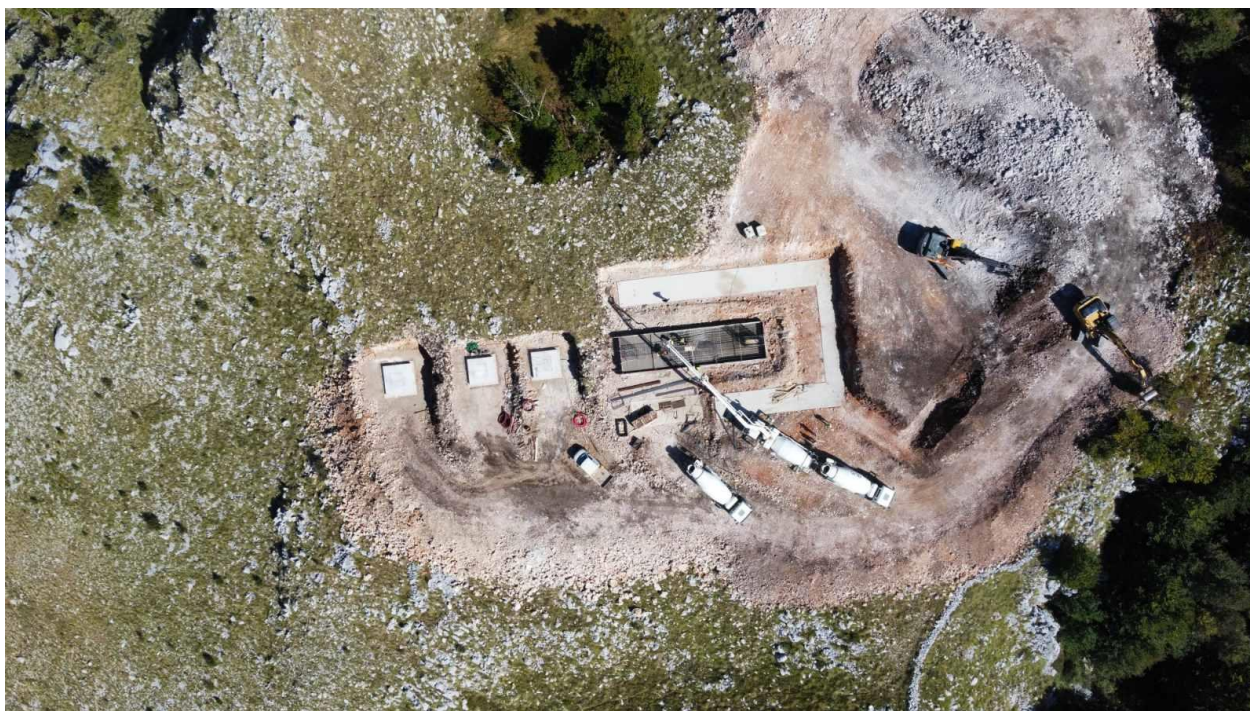
Figure 10-11: The top station (casting of the foundation slab) and foundations S17 to S19
