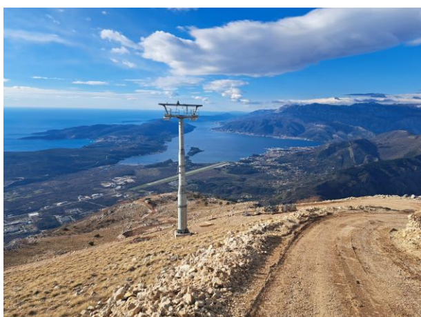
Tower W16 and towers S17 to S19
