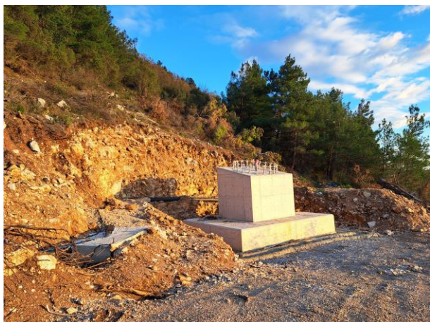
Towers S5 and S6
