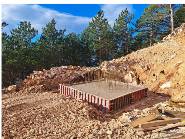
Towers S12 and S13
