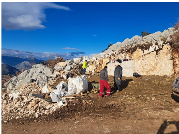
Towers S14 and S15
