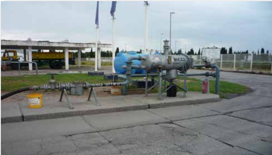
Podgorica Airport: 'Fuel Farm'
