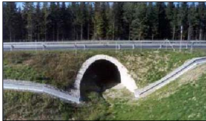
Arch culvert with fence for large mammals and lipped wall for amphibians (FHWA/US DOT, 2002)
